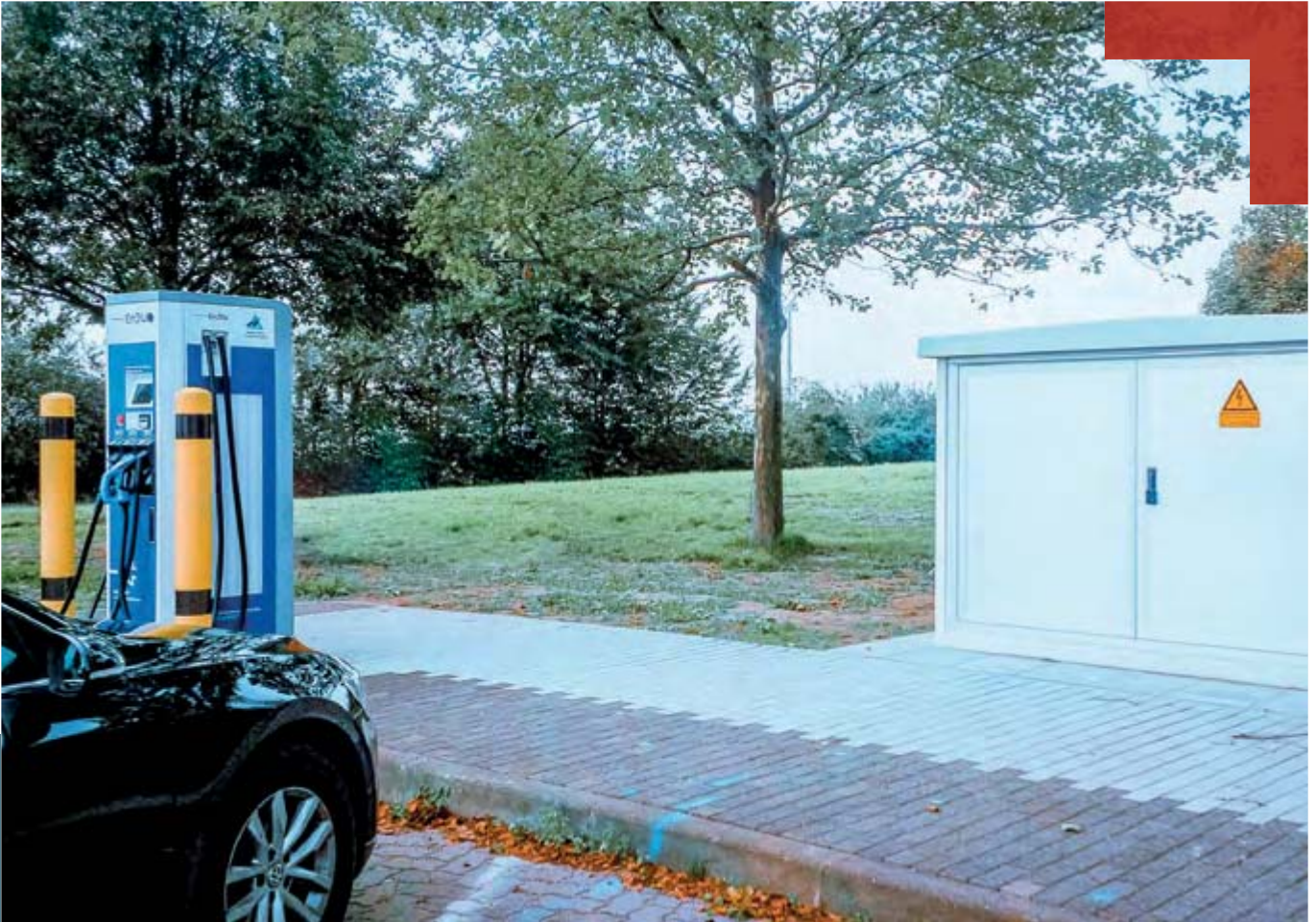
A station in a public space providing electricity for car charging.
