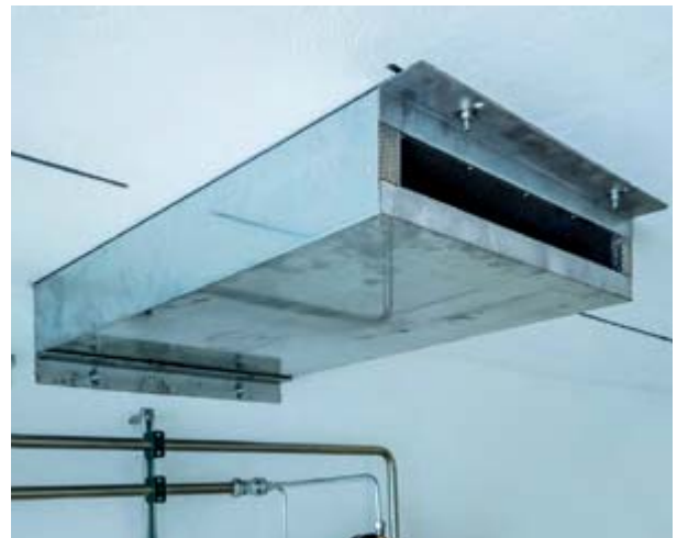
A soundproofed sheet duct.
